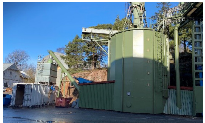
The picture shows a dust silo with a modified transport system, resulting in fewer briquettes for incineration.
